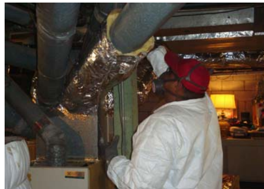
Wrapping the duct-work in Janice's basement will result in overall energy savings.
